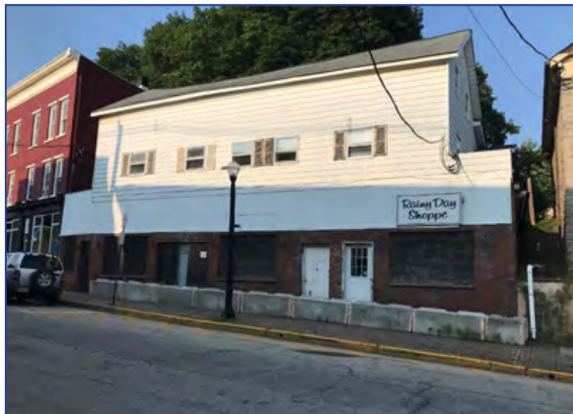
Image 111. Deteriorating condition of the former Rainy Day Shoppe building at 12-18 Main Street.
