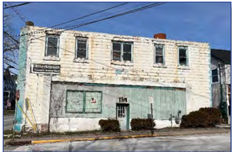
Images 106 and 107. The Former Blacksmith Cycles building is prominently located at the intersection of Bank Street (State Route 23) and Newton Avenue.
